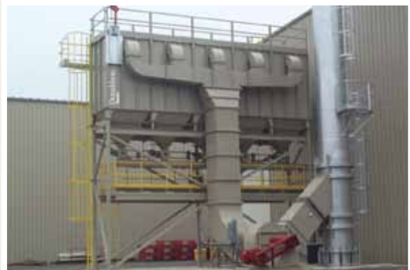
405MBT8 at a brick manufacturing facility
