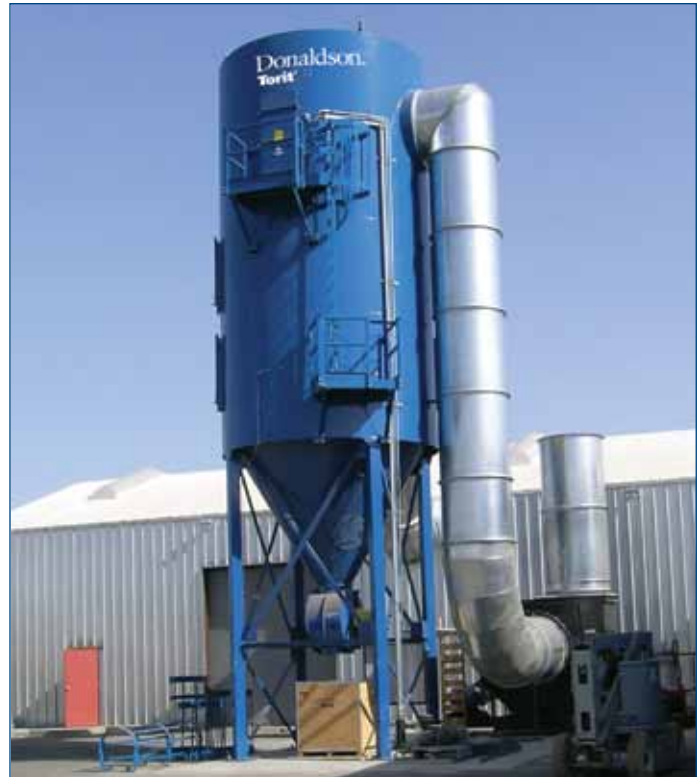
The Dura-Life bag filters in this Donaldson Torit RF Baghouse collector provide longer life and lower emissions at this Midwestern soybean processing plant.
